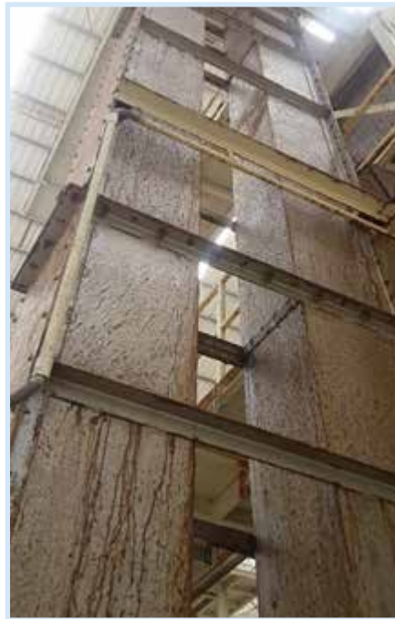
Closed system - cannot be cleaned
